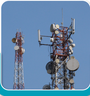
ANTENNA BASE STATION
