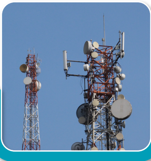
ANTENNA BASE STATION
