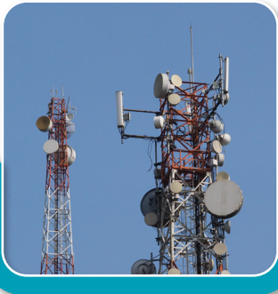
ANTENNA BASE STATION
