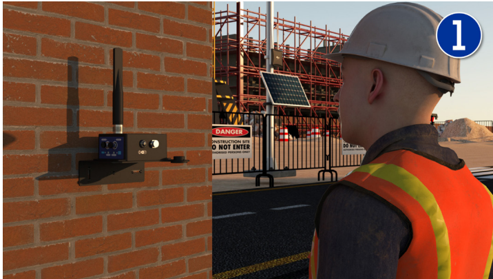
Caption1: After installing the Alpha-Inc inclinometer , the field operator can check at any moment if the sensor is working properly.
